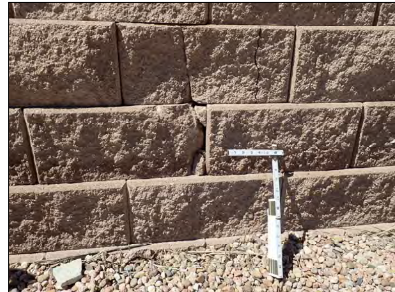
Splits in CMU Block at Sta. 3+45
