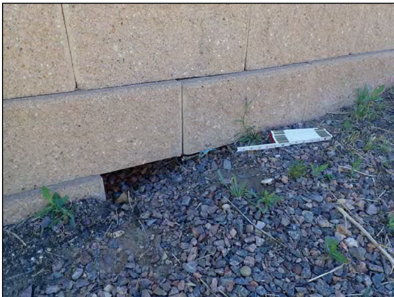
Area of Undermining at Sta. 11+79
