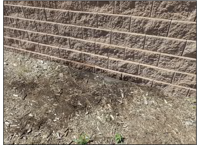
Moisture Staining at Wall Facing and Area of Saturated Ground at Toe of Wall at Sta. 12+57
