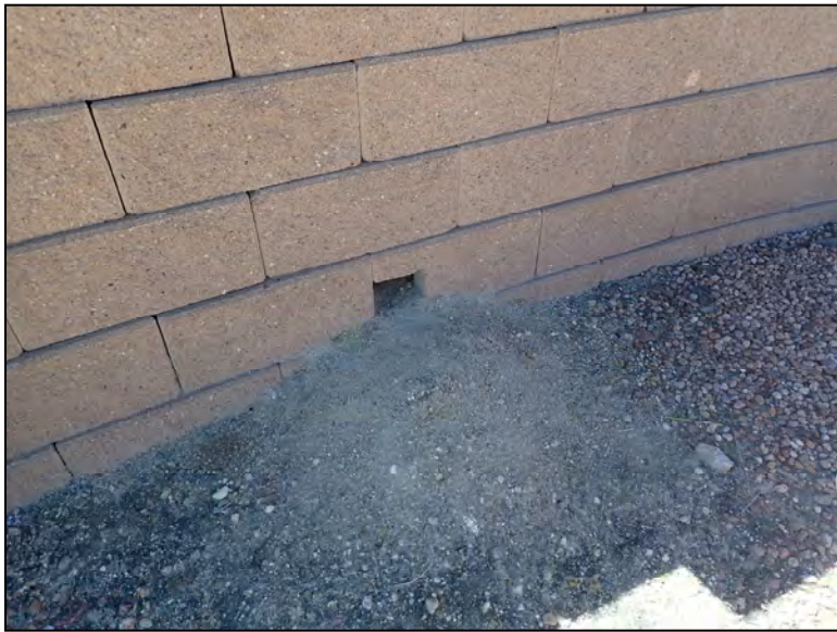
Backfill Loss Through Improperly Installed Weep Hole at Sta. 11+30
