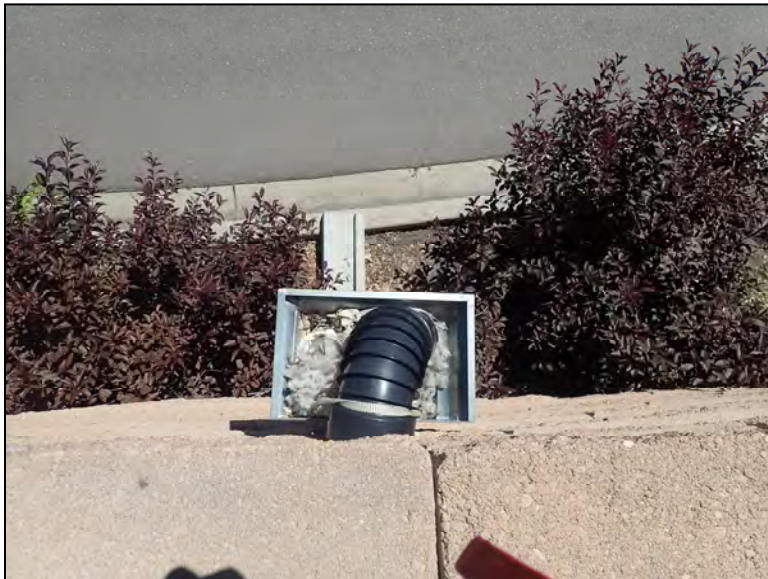
Partially Obstructed Drain at Weep Hole at Top of Wall at Sta. 1+86
