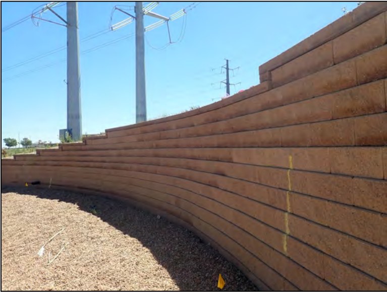
Area of Moisture Staining on Wall Facing at East End
