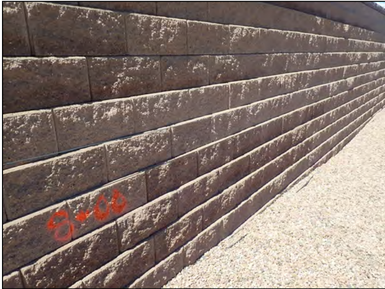
Area of Moisture Staining on Wall Facing at Sta. 8+00
