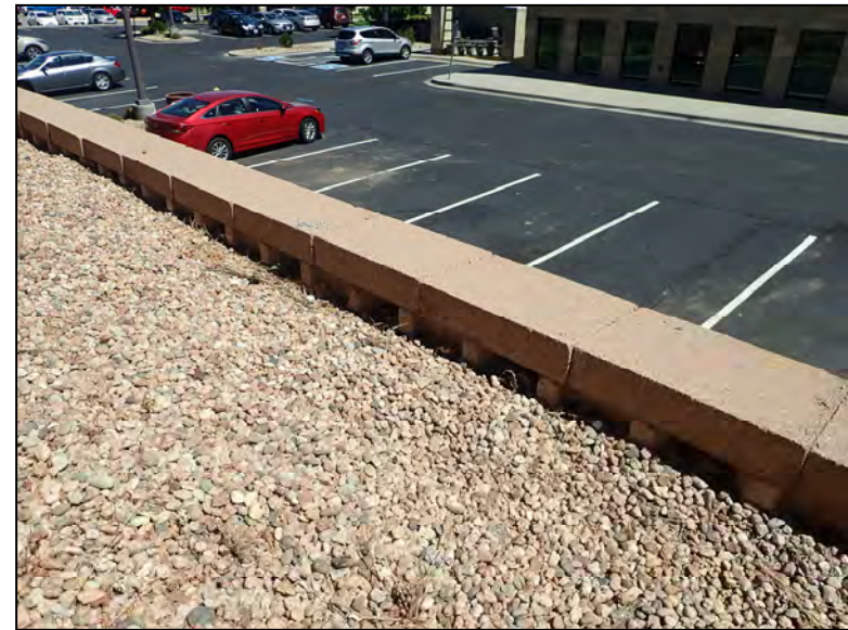
Typical Exposed Top Course of Masonry Block at Top of Wall
