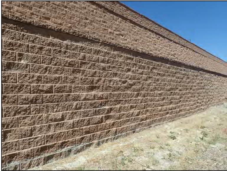
Intermittent Areas of Mortar Residue on Edges of Blocks East of Sta. 14+55
