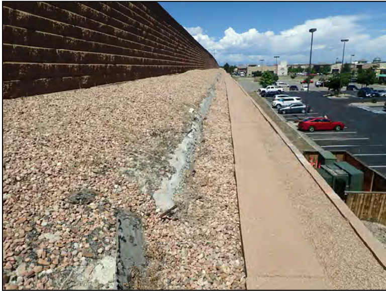
Typical Exposed Shotcrete Wall with Exposed Reinforcing Steel at East End of Wall
