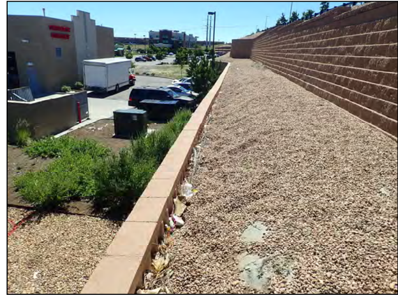
View of Bowed Area of Wall Facing at Sta. 4+90
