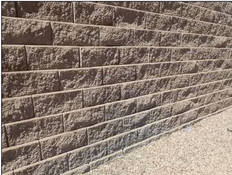
Typical Mortar Residue on Wall Facing
