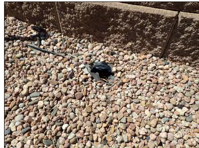
Obstructed Weep Hole at Sta. 7+51
