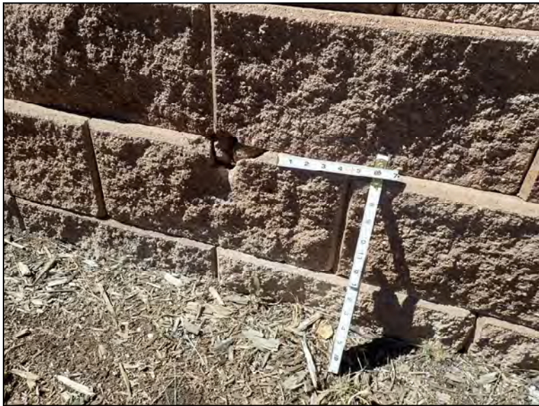
View of Spall in Wall Facing at Sta. 13+14
