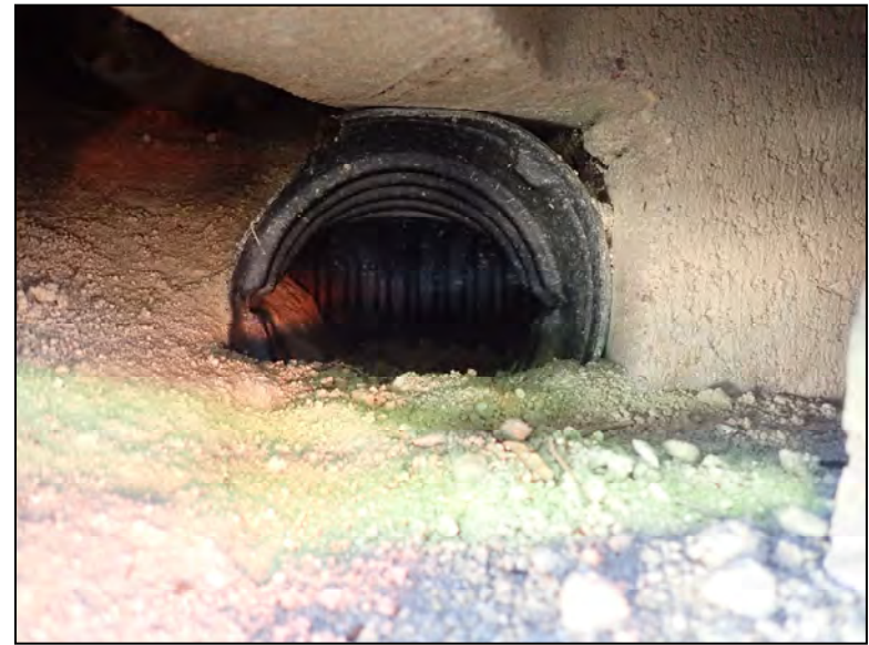
View of Improperly Installed Weep Hole at Sta. 11+30
